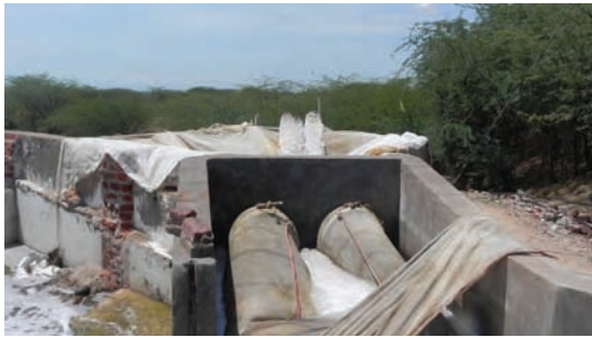
GAqP-Filtration of water at intake
